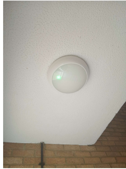
Lighting (Standard and Emergency Lights)
